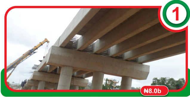
Construction of flyover from Ijigbo (Union Bank) to Okeyinmi (First Bank), Ado-Ekiti
